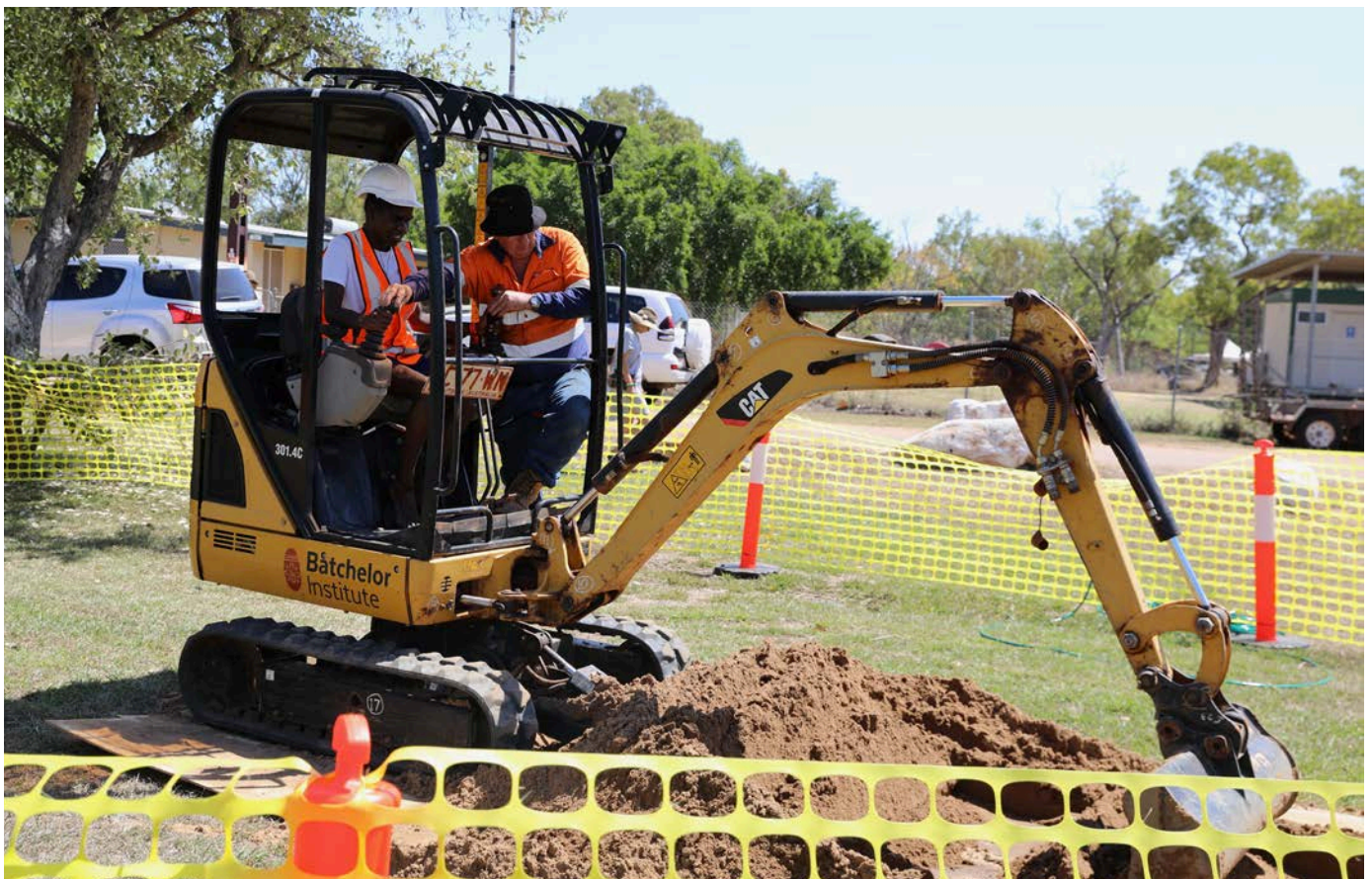
Civil Construction students learn machinery operations, Barry Whalan, VET Lecturer Resources and Infrastructure
